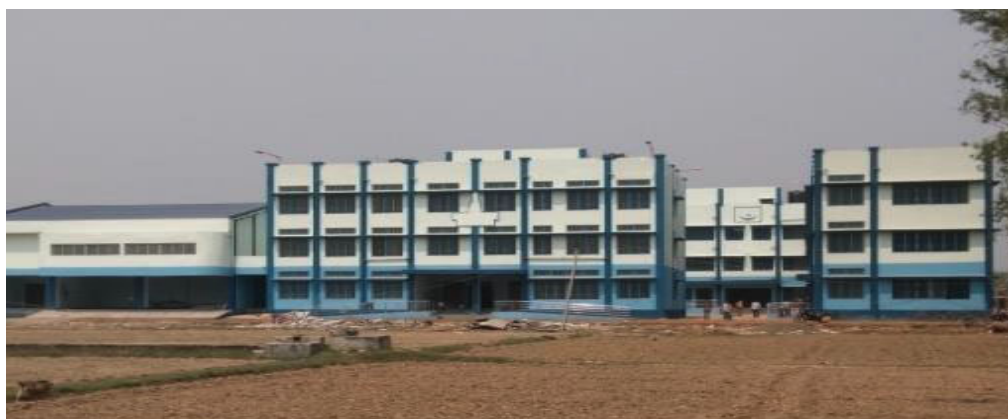
Figure 2.1.12: Under construction Madrasha and its hostel buildings at BSF Keshpur in Paschim Medinipur District
